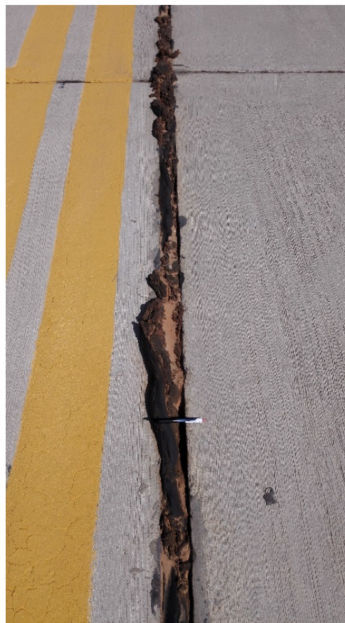
Figure 8. Joint sealant damage due to heat.
