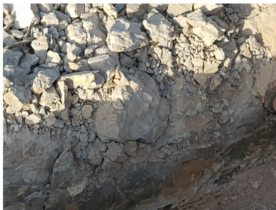
Figure 15. Excavated test pit showing fractured concrete.
