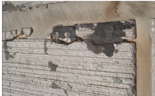
Figure 6. Deformed joint sealant crack patching.
