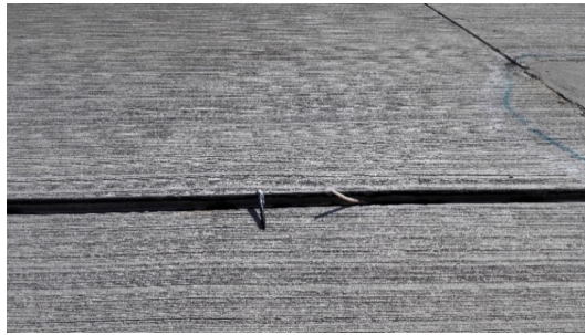
Figure 9. Curling of slabs and poor sealant condition.
